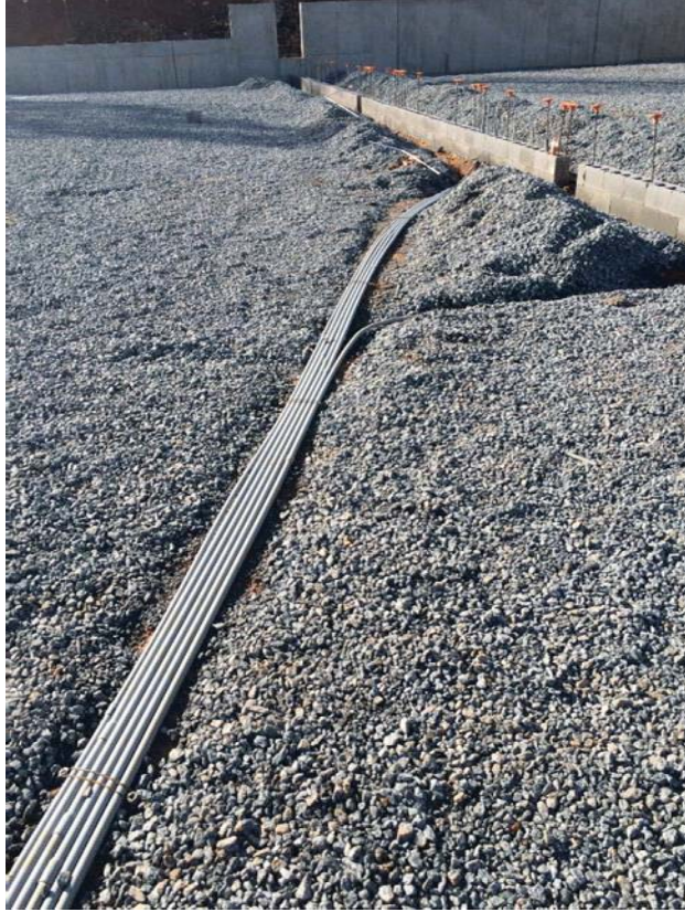
Under Slap Electrical
