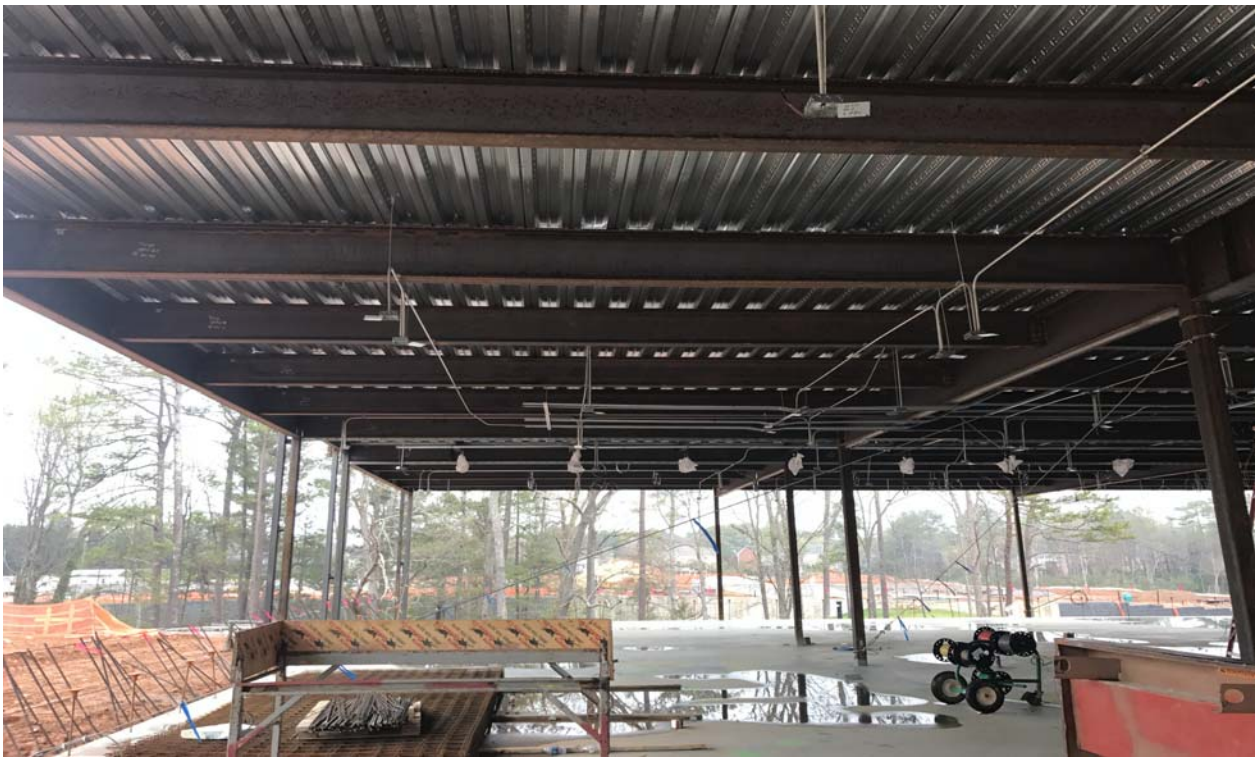
Main Level Overhead Electrical
