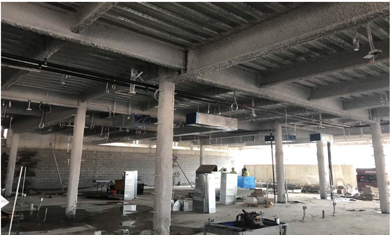
Lower Level HVAC
