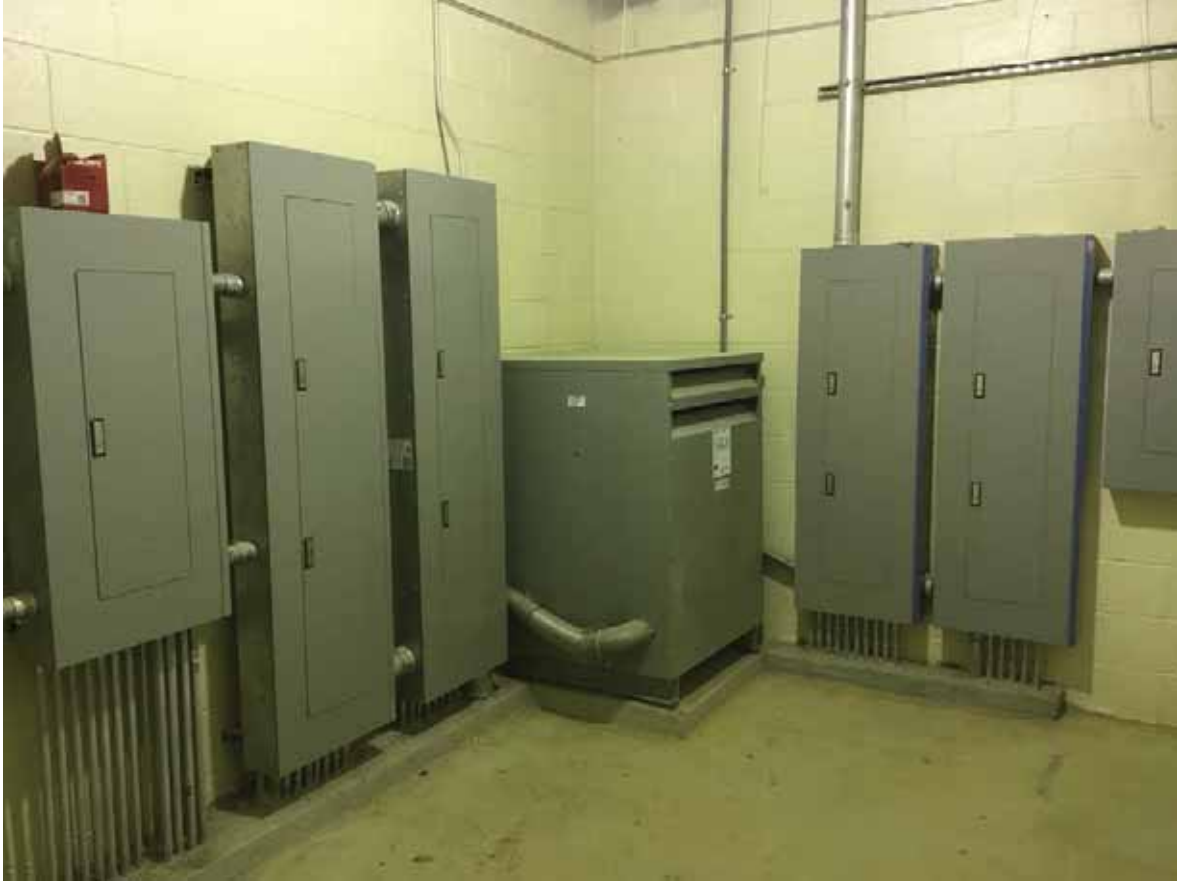
Electrical room on lower level.
